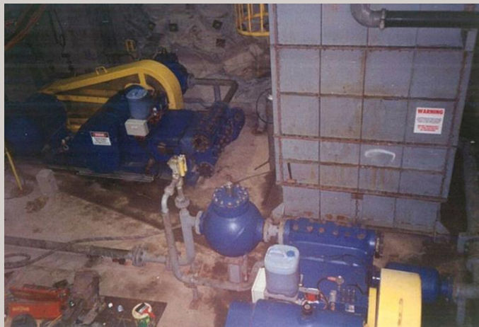
Underground Pump Station at KCGM's Chaffers Shaft
